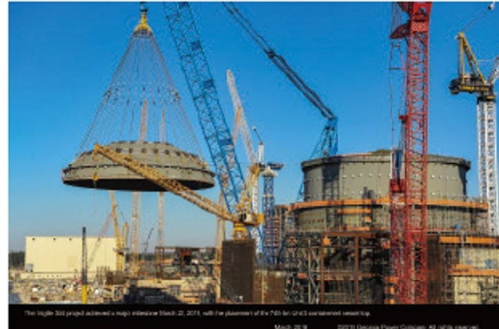
Containment Vessel From IHI Photo provided by Georgia Power Company
