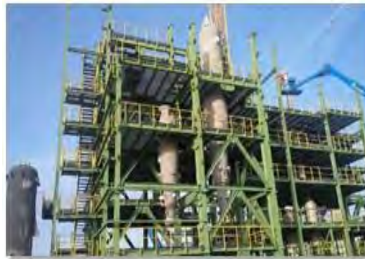
PRENFLO biomass gasification Dunkerque, France Biomass-to-Clean Jet Fuel
