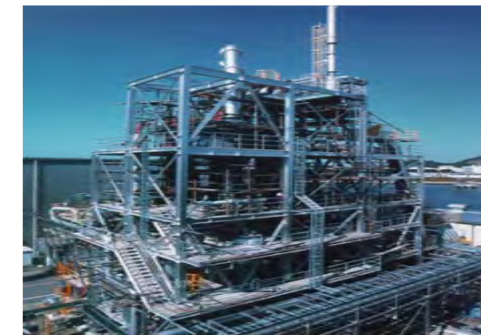
HTW MSW gasification Niihama, Japan waste-to-energy
