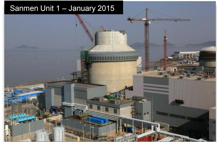
Photo © Sanmen Nuclear Power Company, Ltd. All rights reserved.
