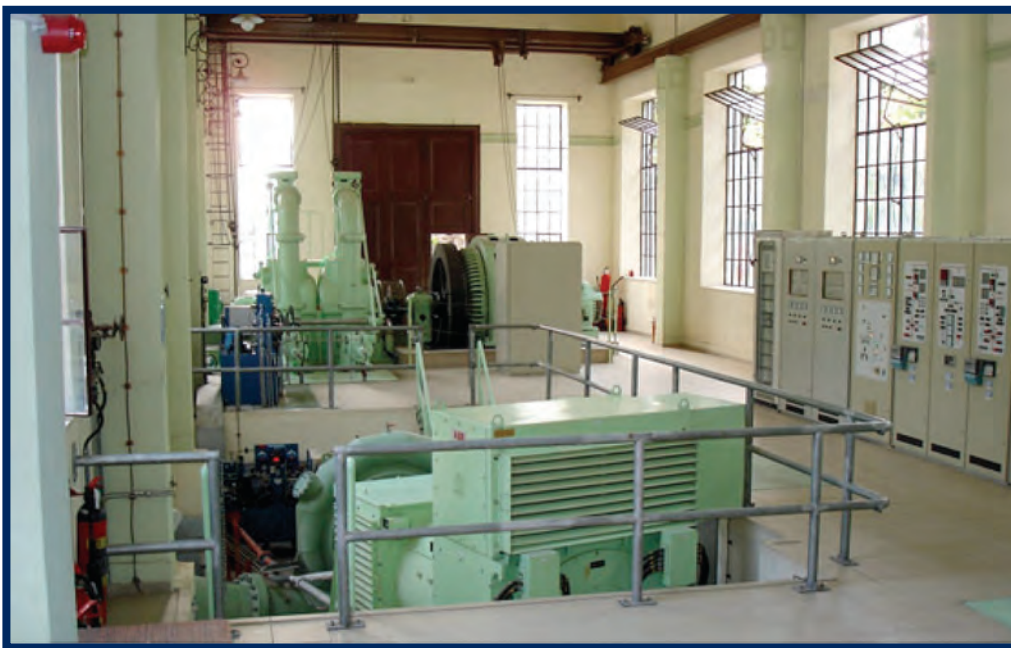
SHPP Achaia-Patra- Glafkos 3,7 MW, in operation since 1922
